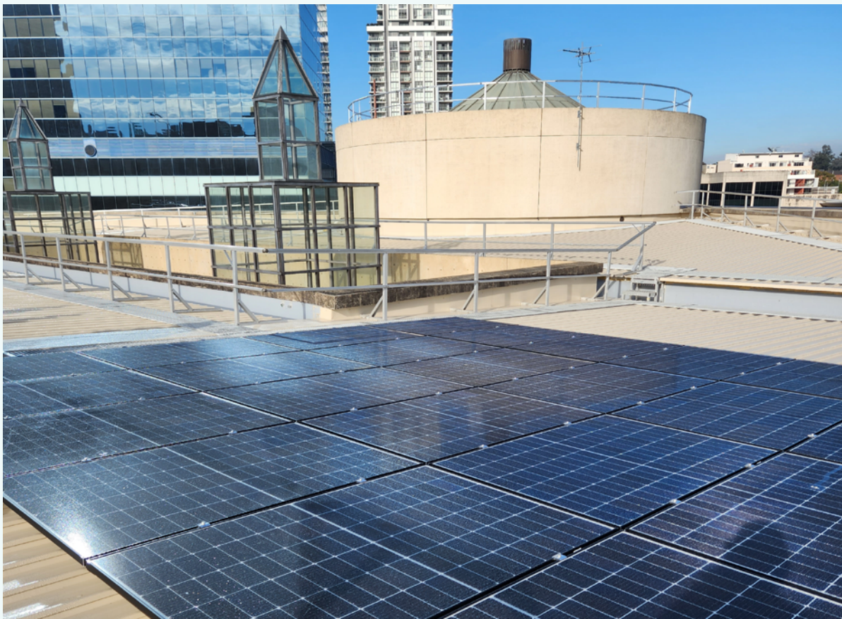
Figure 1: Paramatta CLC solar panels – Photo: Ventia, used with permission
